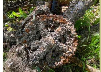
Zebra mussels coat and damage infrastructure in the Great Lakes Region.
